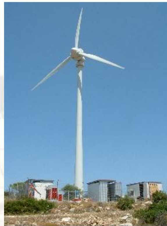
General View of wind-hydrogen installation
